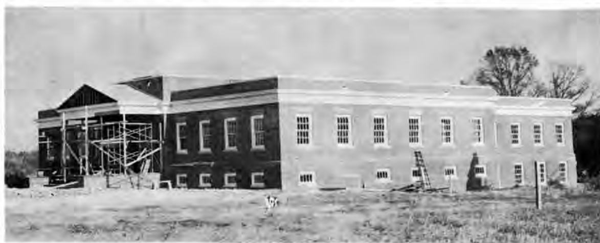
BOWIE'S NEW LIBRARY , located southeast of the administration building, will soon be ready for occupancy.
